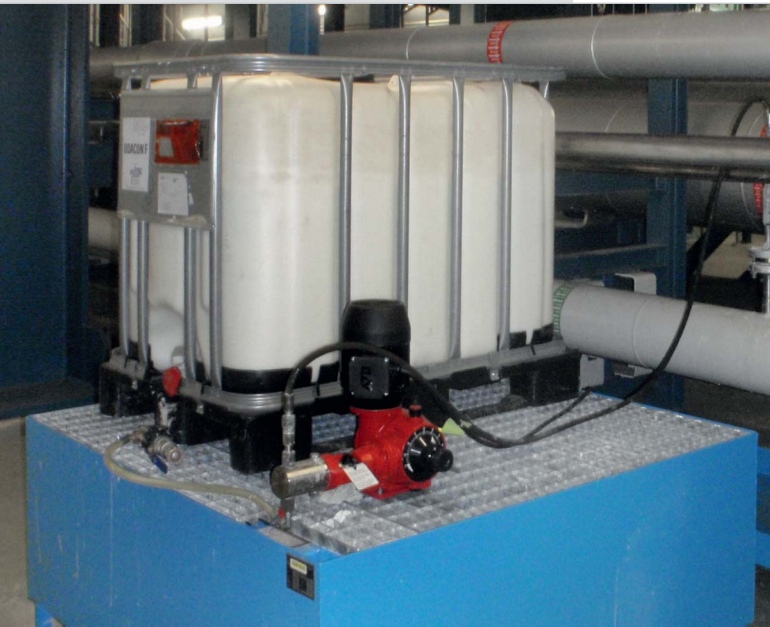
ODACON® dosing in main condensate with high pressure piston pump
